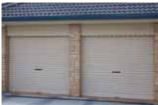
Examples of not approved garage doors
